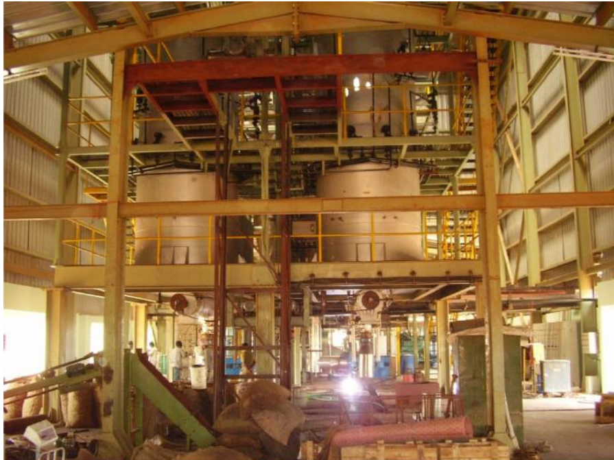
BMC GASIFIER PLANT(1700Kgph)
